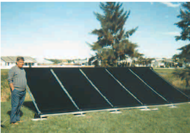
Solar pool panels—ground mounted.
