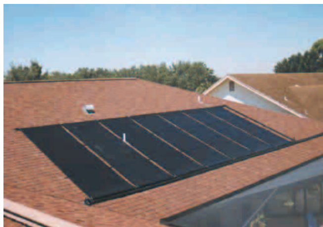
Solar pool panels—roof mounted.
