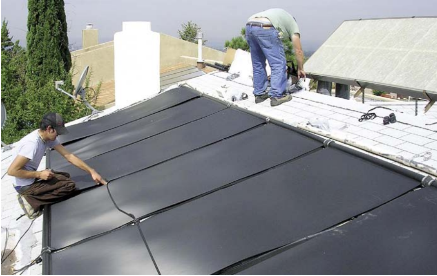
Don Keefe and Jason Urias of AAA Solar in Albuquerque, New Mexico, install a pool system. Note the strapping that secures the collectors to the roof.
