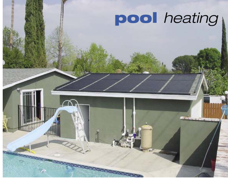
Roof-mounted solar collectors for pool heating are unobtrusive and a highly effective use of space.
